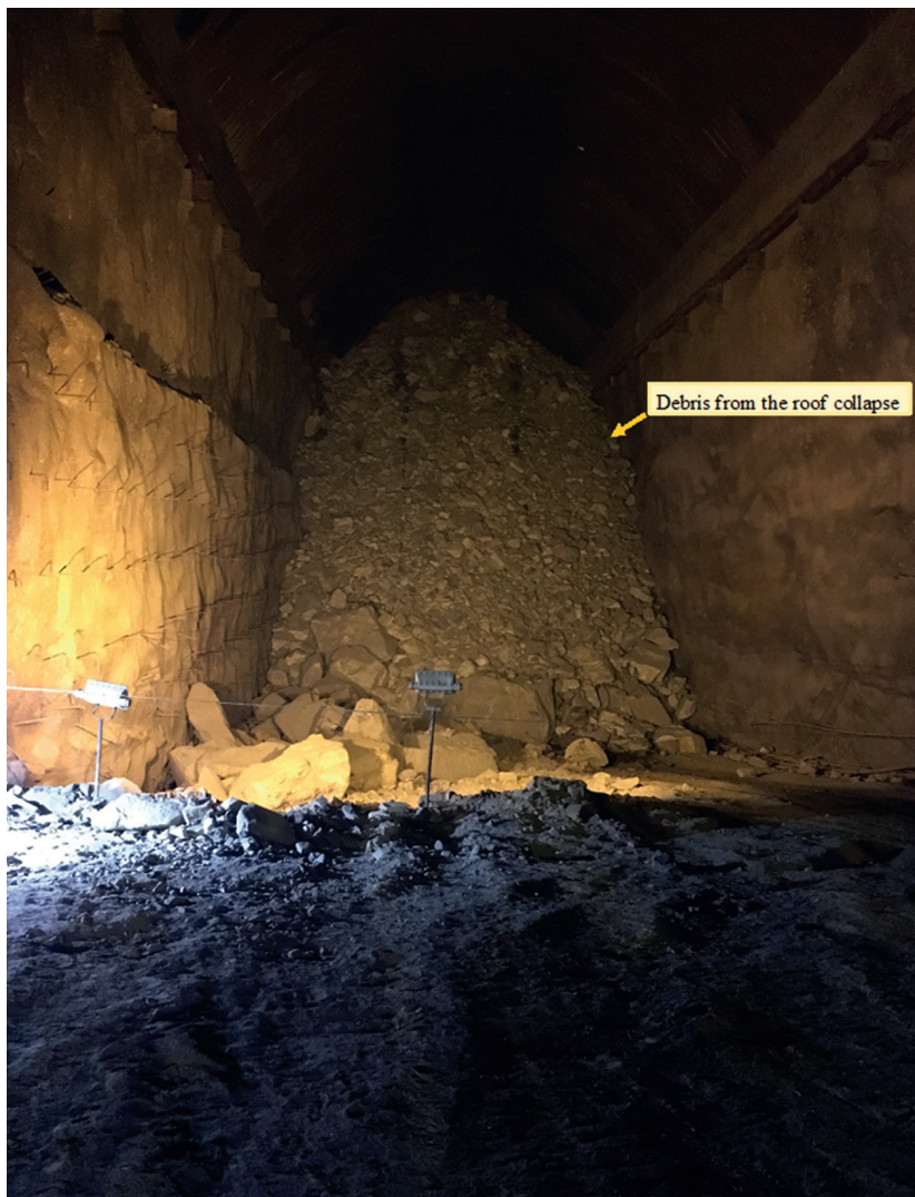
▲ The ceiling in the main tunnel collapsed, completely blocking the tunnel and forming a cavity of unknown size and shape above.
