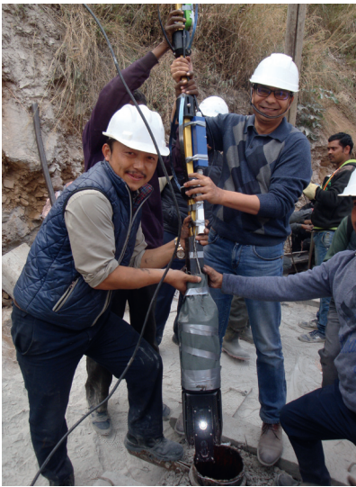
▲ The on-site team prepares to lower the CMS into the borehole, a process that took several hours.
